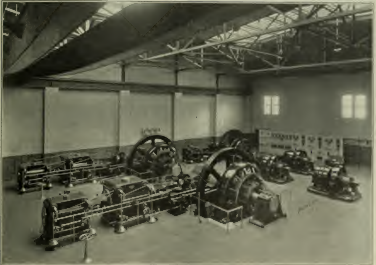
FIG. 11. THE ENGINE ROOM
